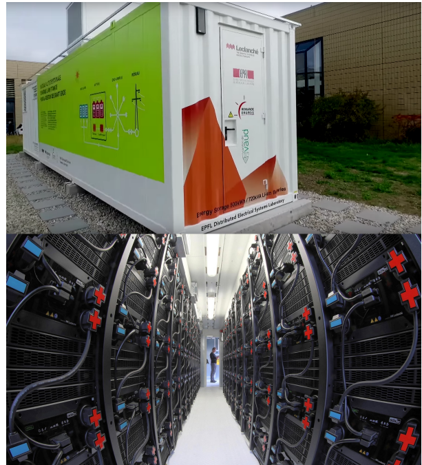
Fig. 7. An outside (top picture) and inside view (bottom picture) of the 720 kVA/500 kWh Lithium Titanate-based BESS used in this experimental work. The system, developed by Leclanché, includes a four-quadrant fully controllable DC/AC converter and a 0.3/20 kV step-up transformer. It is hosted in a temperature controlled container (picture of Alain Herzog, EPFL).
