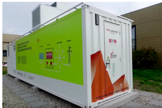
Fig. 1. The 720kVA/500 kWh grid-connected BESS installed at the Swiss Federal Institute of Technology of Lausanne (EPFL) used to validate the “dispatchable feeder” concept.
